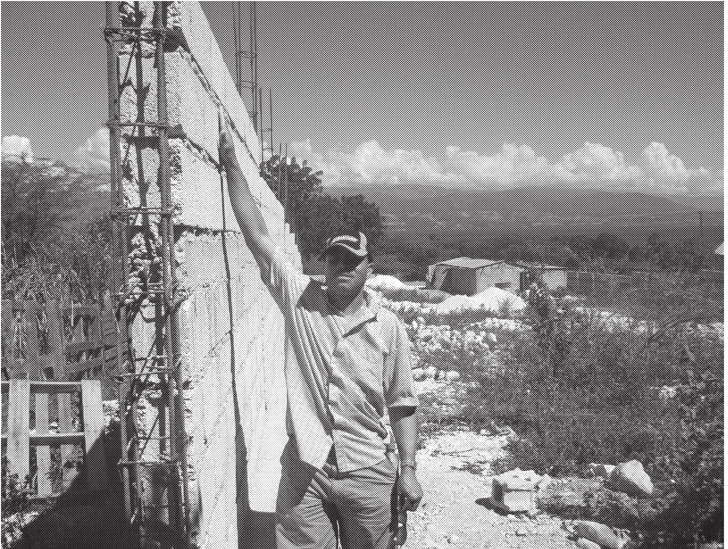
Jean Volcy, an elder of the Strathmore Boulevard Church of Christ, stands beside a portion of the security fence that is part of the work under construction in Fond-Parisien, Haiti. See his report on the progress this Haiti Mission on page 14.
